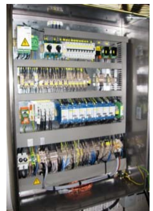
Switch Box with digital CAN Bus modules
