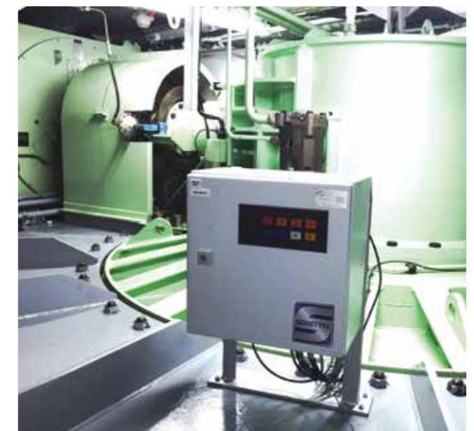
Data collected in the engine room using sensors enables remote maintenance.
